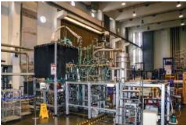
Figure B.1.16: Gyrotron set up at ITER-India Gyrotron test facility.
