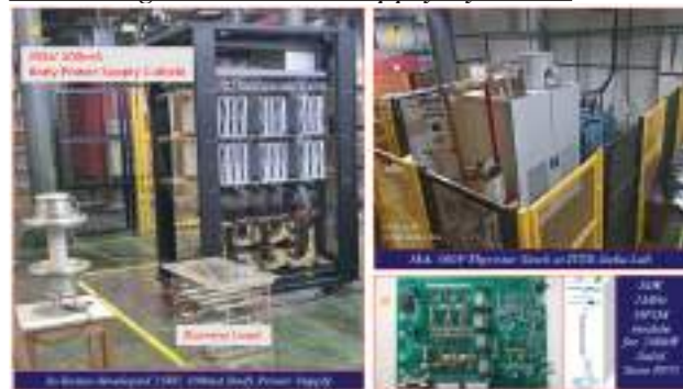
Figure B.1.19: a) Integrated operation of 25kV body power supply, b) thyristor stack development & c) prototype of 3kW HFIM modules for 200kW RFG.
