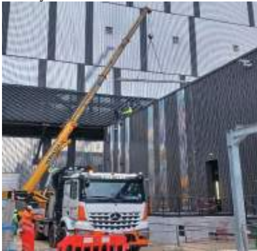
Figure B.1.8: First delivery from INOX in cryo-bridge.
