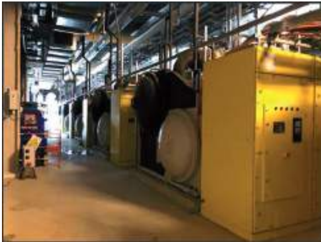
Figure B.1.5: Water cooled chillers.
