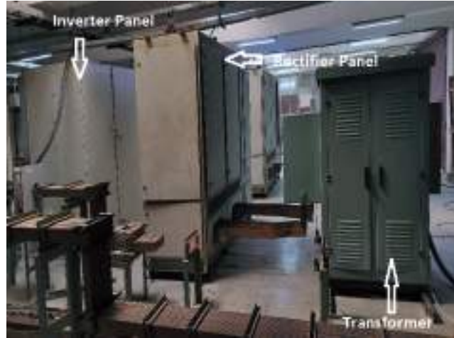
Figure A.3.37: Power Supply, inverter Panel, rectifier panel and transformer.
