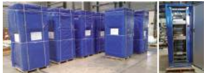
Figure B.1.4: I&C Cubicles delivered at ITER site.
