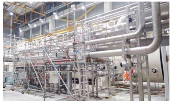
Figure B.8 Installation of warm lines and cryolines underway at ITER site
