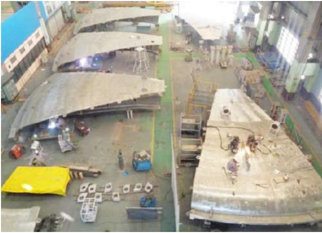
Figure B.2 Manufacturing of Top Lid segments nearing completion at Hazira, India
