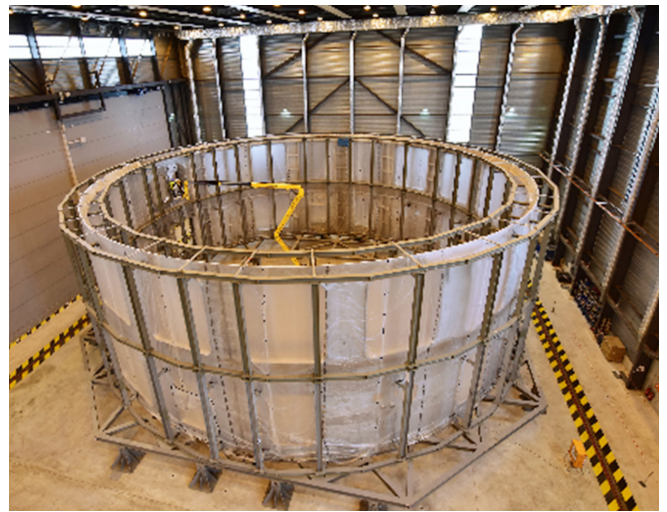
Figure B.1 Cryostat Lower cylinder completed in the workshop at ITER site
