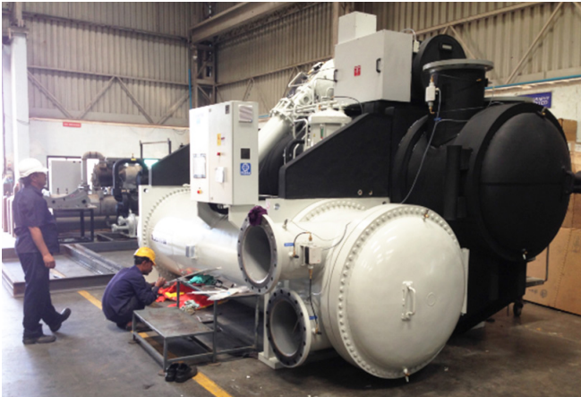
Figure B.2 One of the chillers shipped and delivered to ITER site
