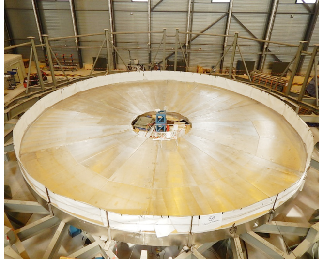
Figure B.2 Cryostat Base Section Tier-1 welding and testing at ITER site workshop
