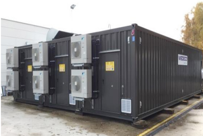
Figure B.3 Ozonation System delivered to ITER site
