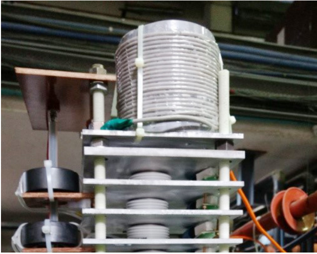
Figure A.1.13 Water cooling Jacket on Electrical Motors of Helium Screw compressors
