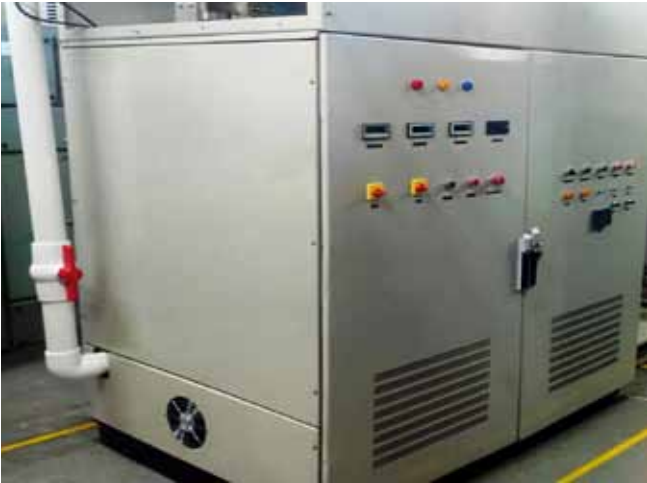
Figure A.3.1.1 The newly installed 10kA/20V power supply in LVPD
