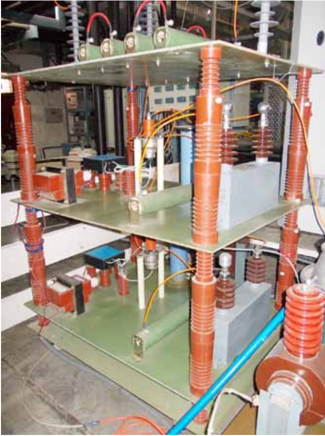
Figure A.1.2.6 70kV Ignitron Crowbar system
