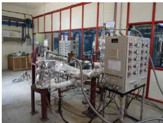
Figure 2.3.2 Pump driven Lead-Lithium loop at IPR
