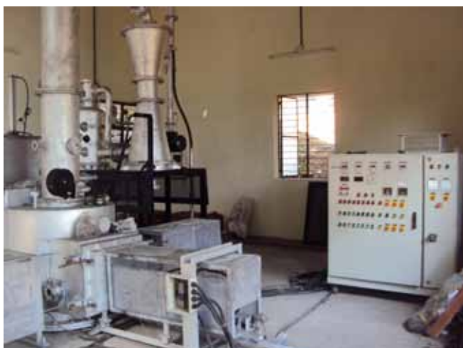
Figure B.1.3.1 : Plasma Pyrolysis System installed at SC-TIMST, Trivandrum
